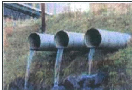
An outfall that is sending water into a storm drain or stream when there has been no rain in the last 72 hours.
